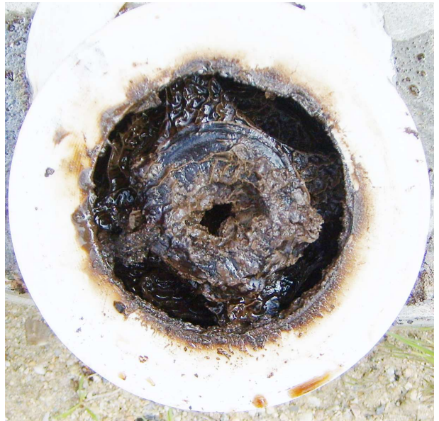
Incrustations in a pipe caused by precipitation of organic material and carbonates
