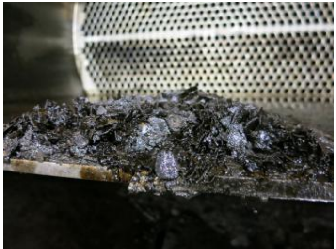
Accumulated scalings inside an evaporator
