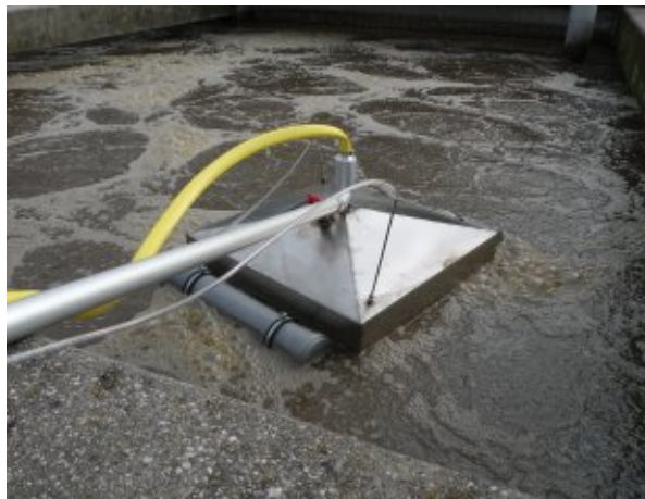
In-house developed gas sampling hood in action at a wastewater treatment plant
